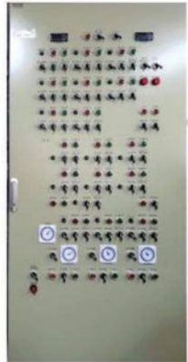
Distribution panel (kontrol ng greenhouse)
